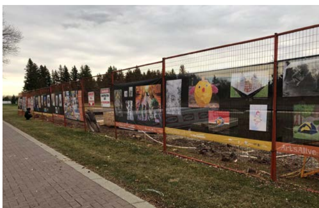
Construction Fencing Public Art Japanese Garden New Community Facility Construction Site Henderson Park
