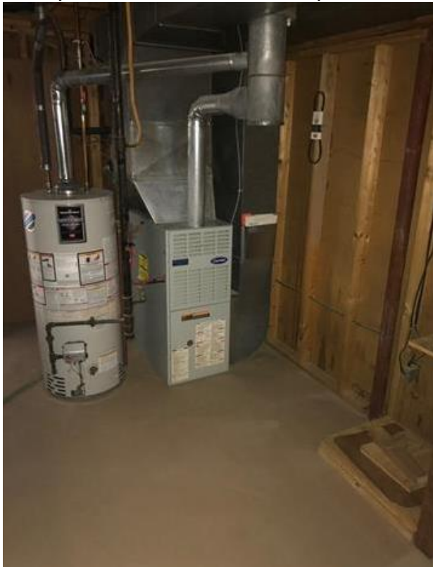
Utility room with furnace – 1 photo
