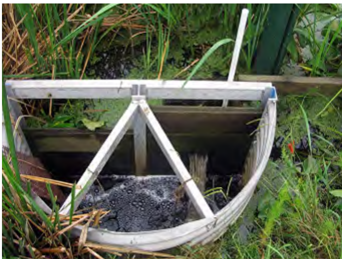
Figure 9. An outlet employing the traditional flashboard riser
