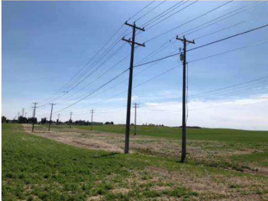
Photograph 9 – Overhead Powerlines Leading to the Substation Facing South Note the pole-mounted transformer. No staining was observed.
