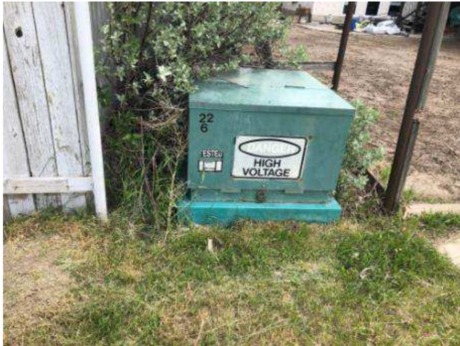
Photograph 27 – Electrical infrastructure along Eastern Boundary of the Property
