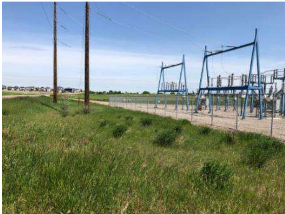
Photograph 2 – Property Overview Facing North-Northeast from Southern Access of Bowron Substation
