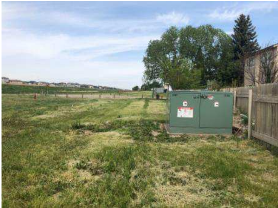
Photograph 26 – Switchgear Located Along Eastern Boundary of the Property Facing North
