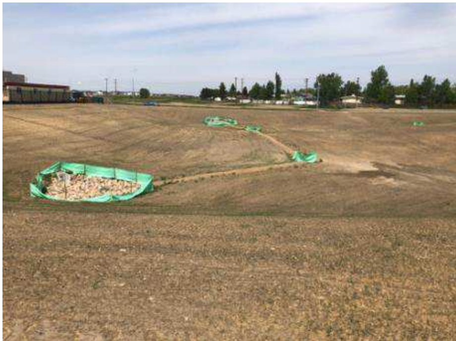
Photograph 36 – Culverts and Drainage System East of the Fire Station Property Facing North
