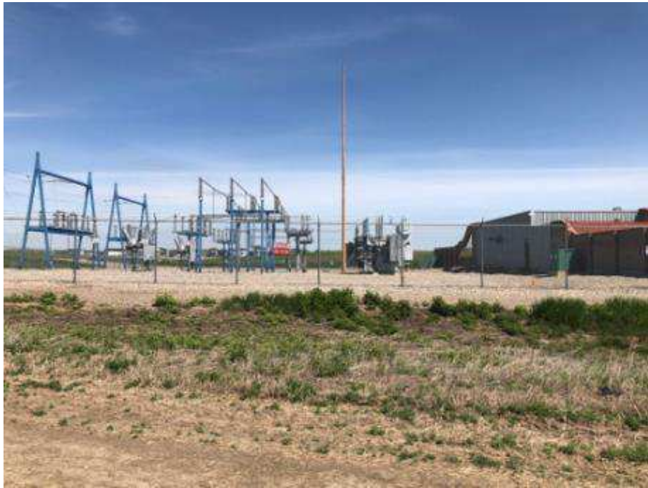
Photograph 7 – Bowron Substation Facing North The substation lot was not accessed.
