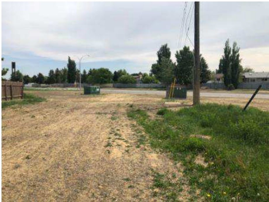
Photograph 30 – Two switchgears Adjacent to Macleod Drive West Facing Southeast The switchgear to the right was manufactured in 2005, and the one in the background was manufactured in 2010.
