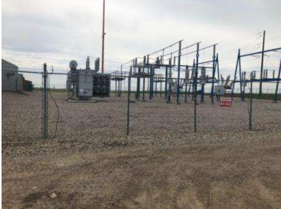
Photograph 10 – Northern Side of Substation Facing South
