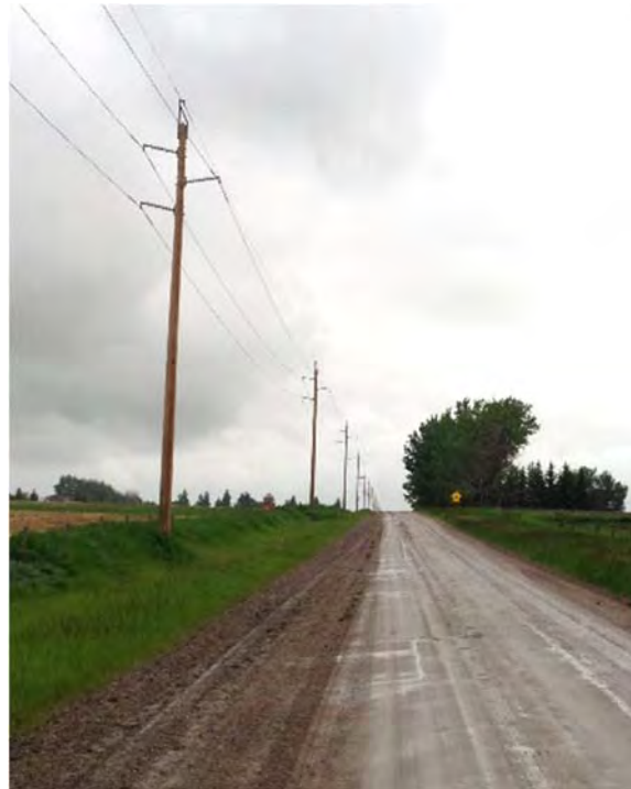
138kV transmission line through SEASP area
